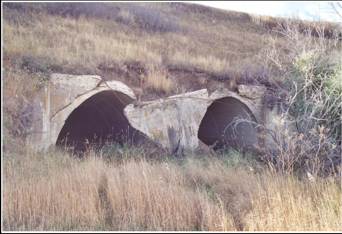
Figure 11. Concrete culvert ruin at the North Montana Line's Box Elder Creek crossing. View to the south/southwest.
