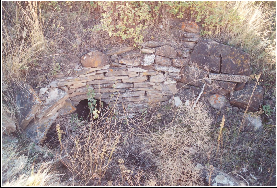
Figure 15. A typical dry-laid fieldstone culvert headwall along the Rainbow-Ryan Road (24CA416). View to the southeast.
