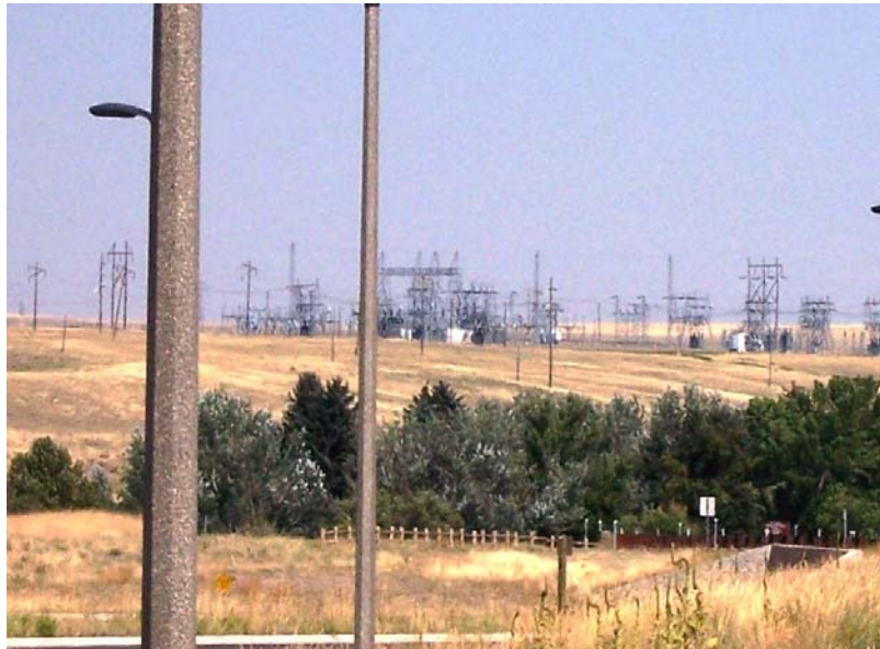
Figure 3-52. Great Falls Switchyard from Lewis and Clark National Historic Trail Interpretive Center Parking Lot
