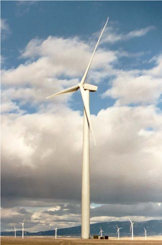
Figure 2-30. 1.5-MW GE Wind Turbines at Judith Gap, Montana
