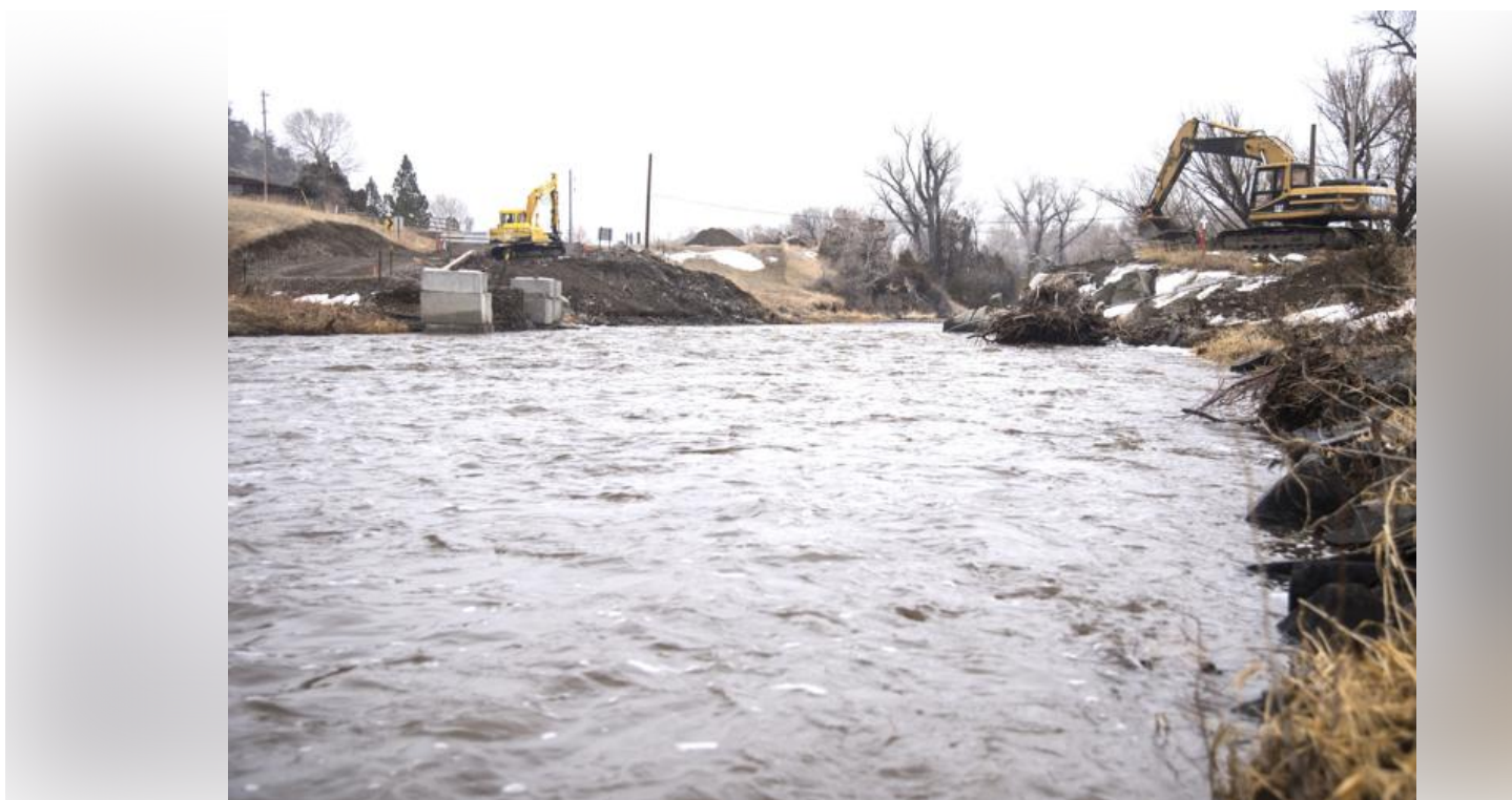
An excavator cleans up the site where a temporary bridge fell into the Shields River on Monday.
