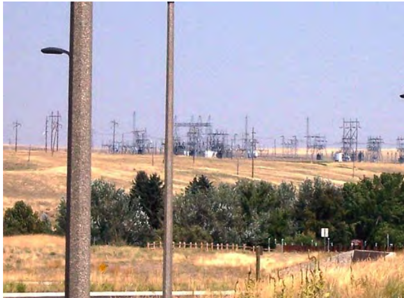
Figure 3-52. Great Falls Switchyard from Lewis and Clark National Historic Trail Interpretive Center Parking Lot
